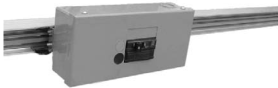
Circuit Breaker installed on Amerlux Busway
