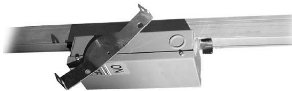
Fused Disconnect installed on Amerlux Busway
